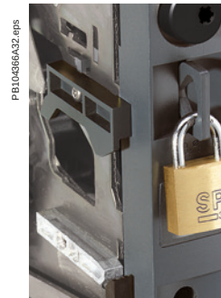
"Disconnected" position locking by padlocks.
