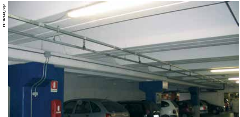
Canalis KBA supplying luminaires nearby sprinklers.
